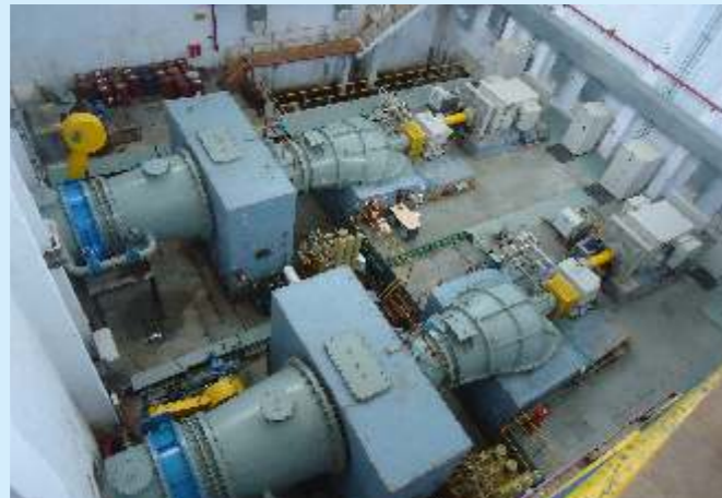
DARNA HEP, 2 X 2.45 MW, HORIZONTAL 'S' TYPE TUBULAR KAPLAN TURBINE
