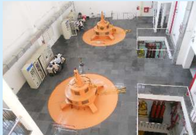
ANKHE KANAK HEP, VIETNAM 2 X 6.5 MW, VERTICAL KAPLAN TURBINE
