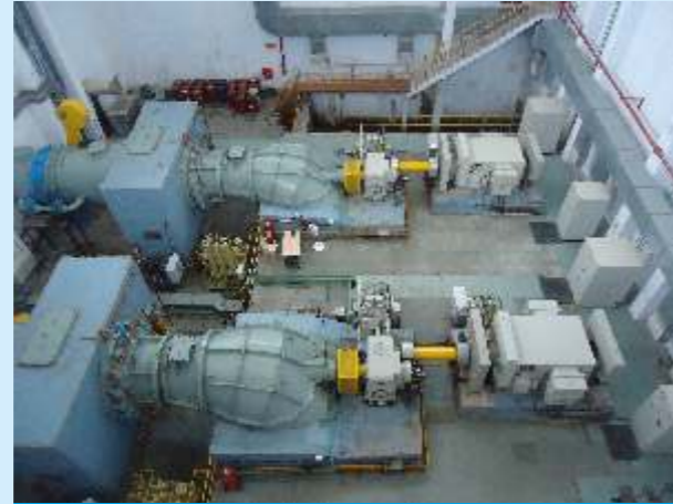
POWER HOUSE INDOOR EQUIPMENT
