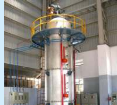
STRESS RELIEVING FURNACE
