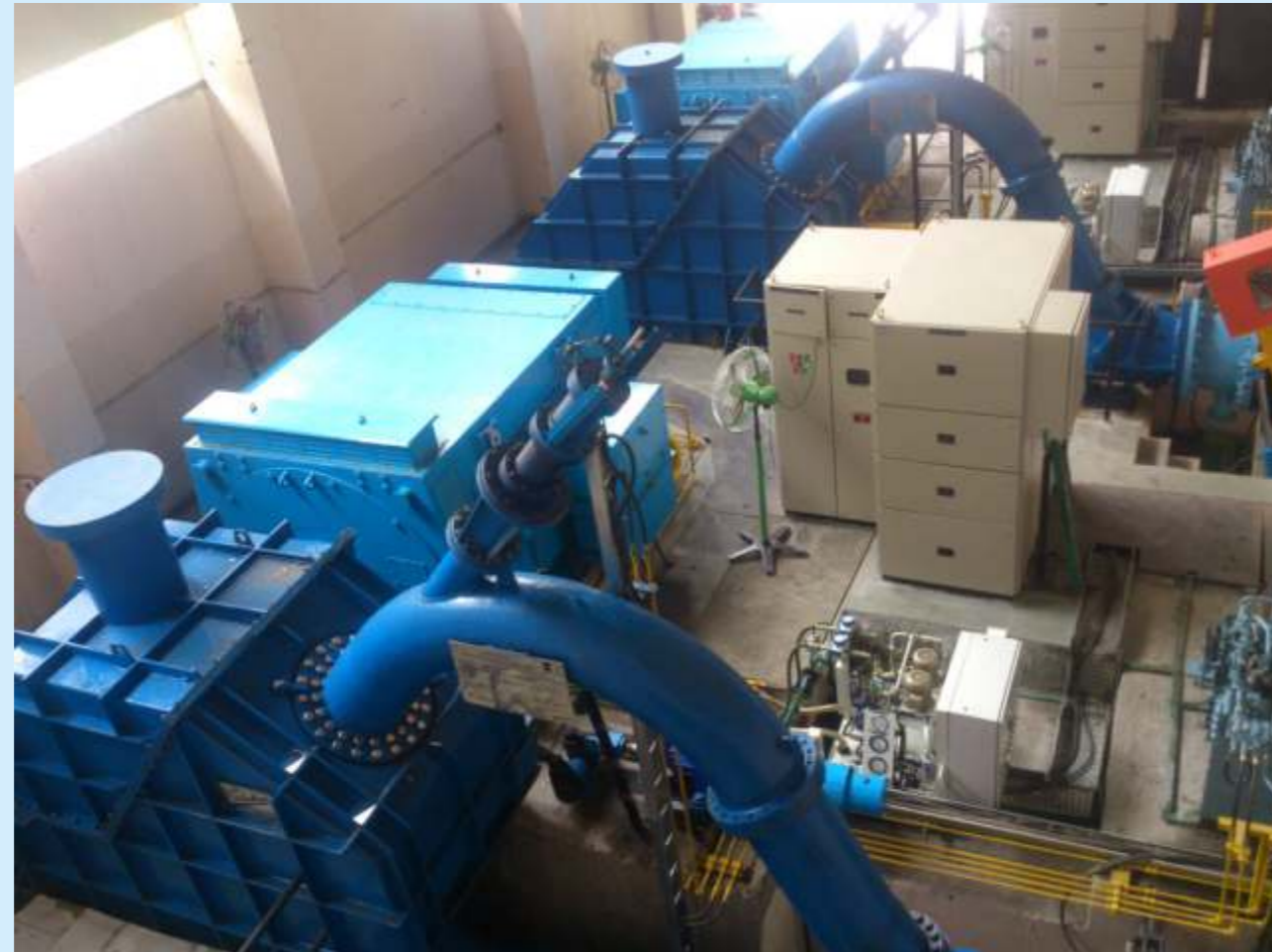
PANWI HEP 2 X 2 MW, TWIN JET PELTON TURBINE
