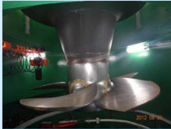
ZHO SUWEI HYDRO POWER PLANT, TAIWAN, 1 X 3607 KW, VERTICAL KAPLAN TURBINE
