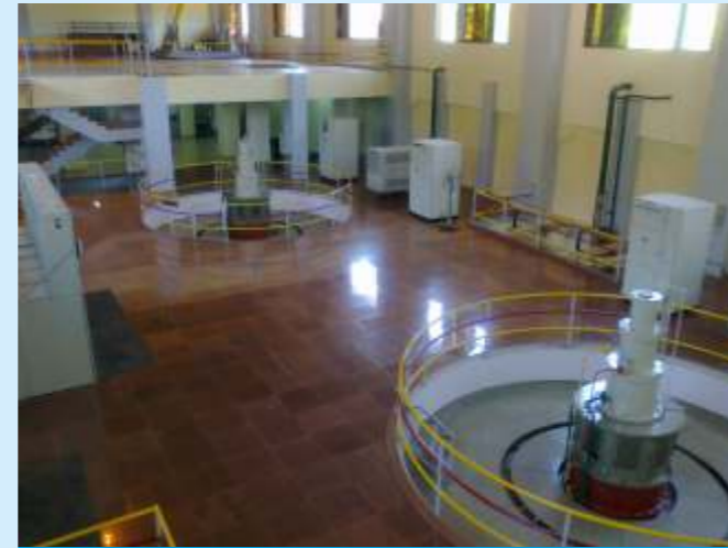
KONAL HEP, 2 X 5.5 MW VERTICAL KAPLAN TURBINES
