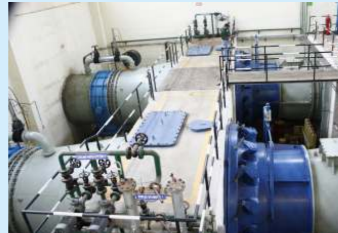
RANNI PERUNAD HEP, 2 X 2 MW, HORIZONTAL 'S' TYPE TUBULAR KAPLAN TURBINE
