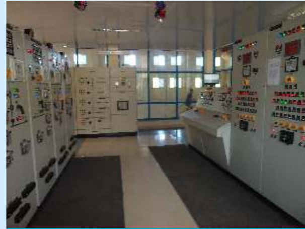
CONTROL & PROTECTION PANELS
