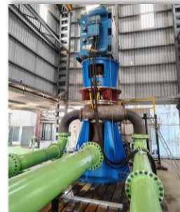
Primary Cooling Pump (PCP) for Pressurized Heavy Water Reactor (PHWR)
